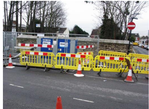
Sewage pumps on Albert Road (Bridge 69) on 30 th January 2017. Network Rail and Thames Water will be working to affect a permanent repair and install a new pile early on Sunday mornings, 19 th , 26 th March and 2 nd April.
