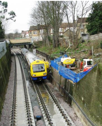
172 006 passes the sewage spilling from the breach with the 12:20 ex Gospel Oak on 11 th March 2017. Photo taken from Bridge 70 (Queen's Rd).
