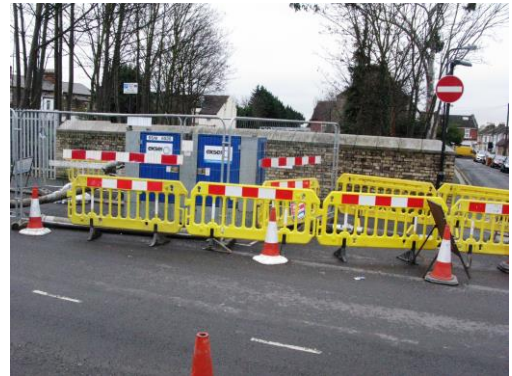
Sewage pumps on Albert Road (Bridge 69) on 30 th January 2017. Network Rail and Thames Water will be working to affect a permanent repair and install a new pile early on Sunday mornings, 19 th , 26 th March and 2 nd April.
