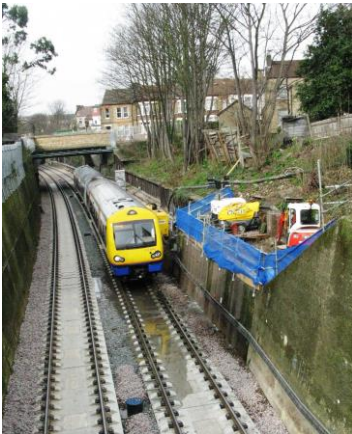
172 006 passes the sewage spilling from the breach with the 12:20 ex Gospel Oak on 11 th March 2017. Photo taken from Bridge 70 (Queen's Rd).
