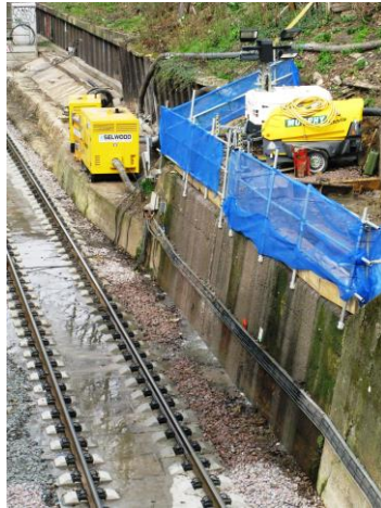
Sewage overflowing onto the track as seen on 11 th March 2017. Photo taken from Bridge 70 (Queen's Road).
