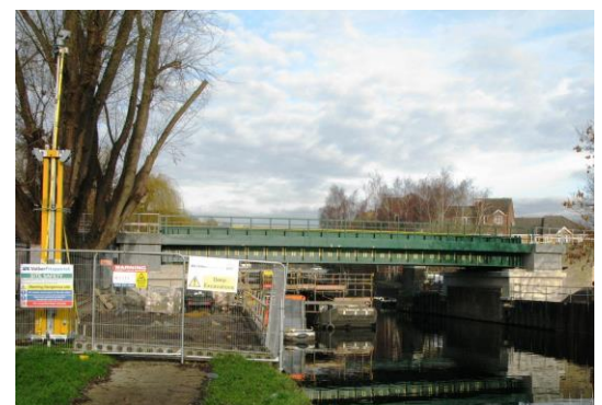
A new Bridge 32 was installed over the Lea Navigation during the New Year holiday. It is still awaiting the electric wires on 2 nd February 2017.
