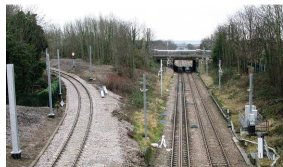
Awaiting the wires at Harringay Park Junction. Harringay Green Lanes station in far distance. The curved track leads to Harringay station and the East Coast Main Line. 2 nd February 2017.
